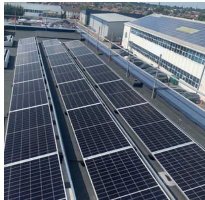
SOLAR PV SYSTEM
