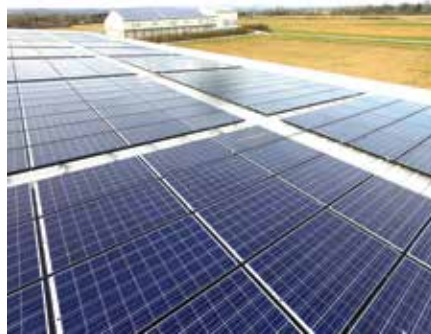
ARRAY - SOLARWORLD PANELS
