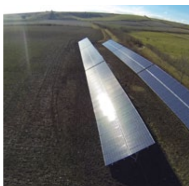
GROUND MOUNT ARRAY
