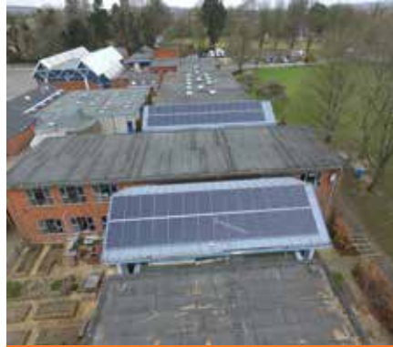
ARRAY 1 - SUNEDISON PANELS
