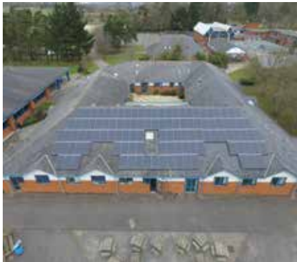
ARRAY 2 - SUNEDISON PANELS
