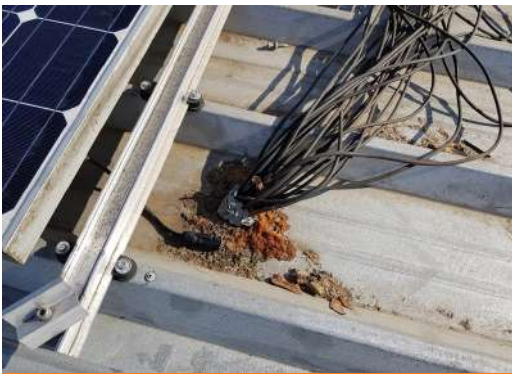
POOR WIRING MANAGEMENT
